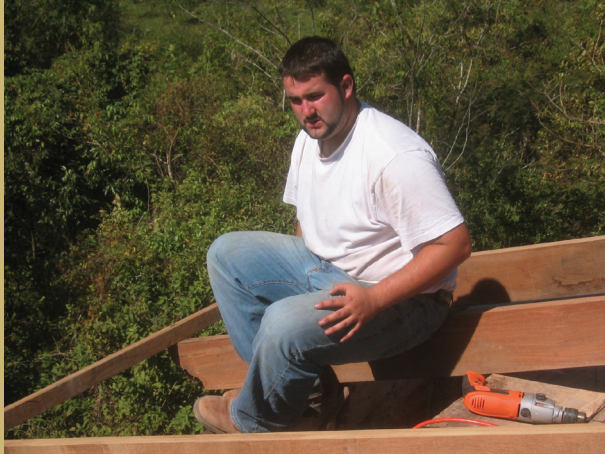
Architecture student Josh Marsh putting the roof on a house at CERENID, Bolivia.
