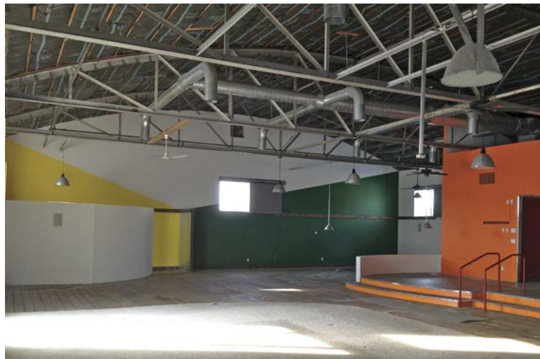
Spacious, with high ceilings, the Logan church awaits interior renovation.
