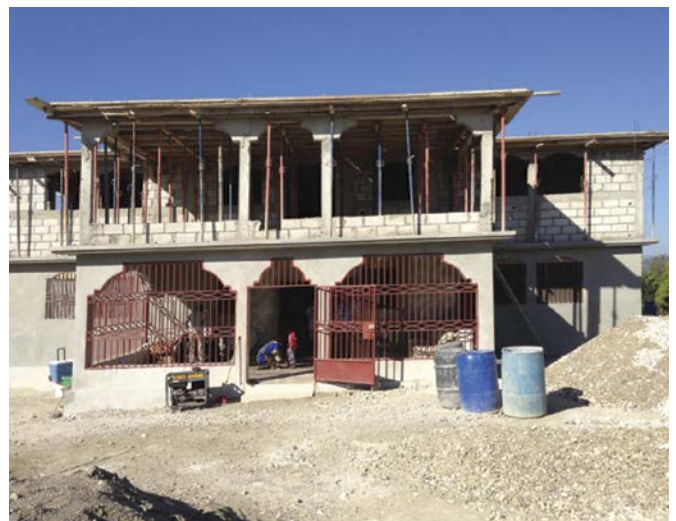
Construction has begun on a new home for orphan girls in Lascahobas, Haiti. The second floor is a guest house for volunteers. The ministry plans to build three more structures like this, then Restore a Child Academy and a vocational training school.
