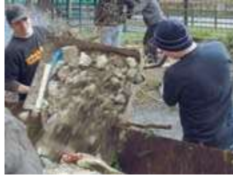
Kyle Verrill, left, and Josh Dezotell working on site to help refurbish the Derry church in Northern Ireland that was built in 1978 by Maranatha Volunteers International.
