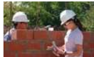
Mark Bugbee and Amy Beisiegel, both from the Berkshire Hills, Massachusetts, church, work on the church construction. It took more than two and a half hours to unload the truck of bricks, one brick at a time.
