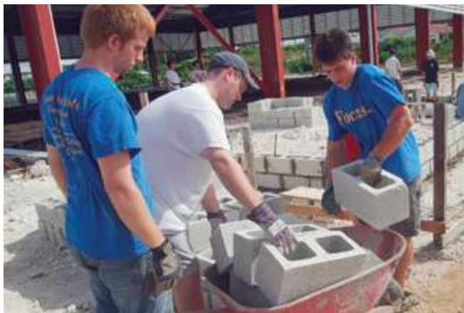
Students and faculty also traveled to Barbados and Nicaragua this year to provide construction labor and spiritual inspiration in Bible seminars.
