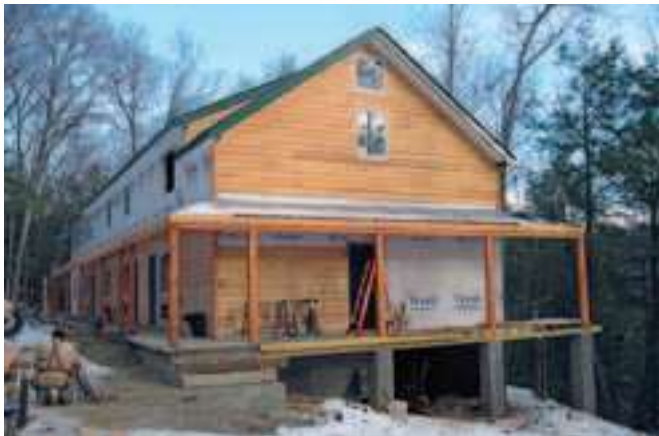
The Montana Lodge is still under construction and is expected to be completed this year.
