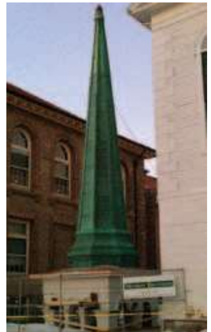
Clinton Spanish church steeple grounded until repairs can be completed.
