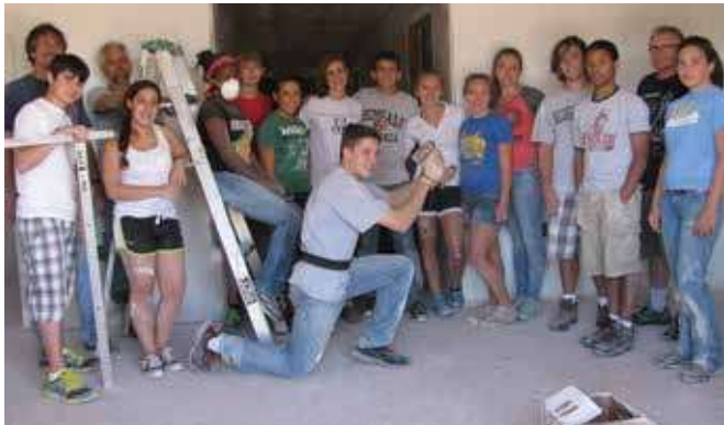
Dressed in work clothes, the team is ready to work, installing insulation, plastic lining, and much more.
