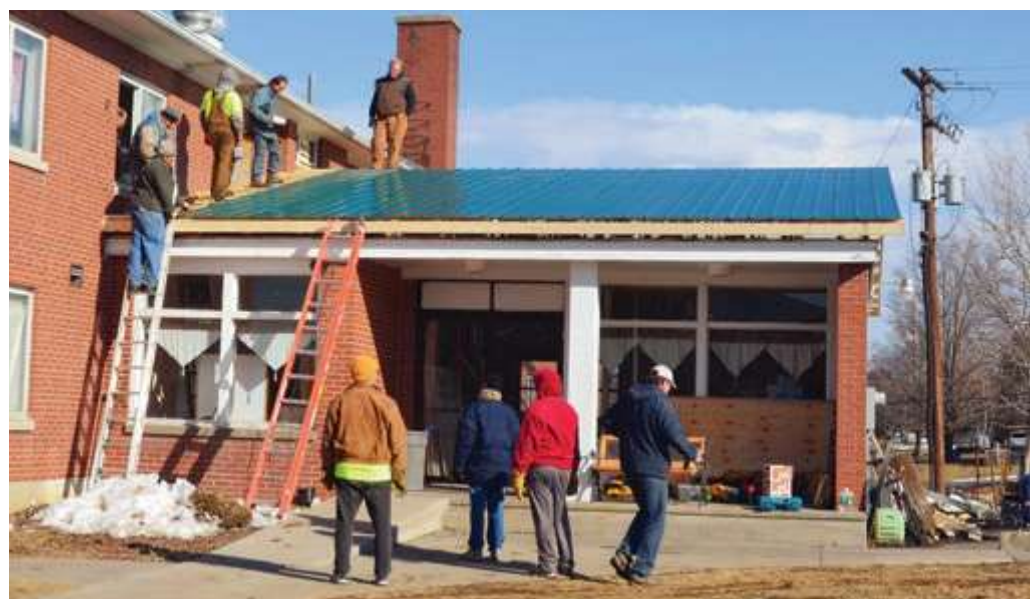
Volunteers finish installing the roof over the boys' dorm lobby and chapel on the Union Springs Academy campus.
