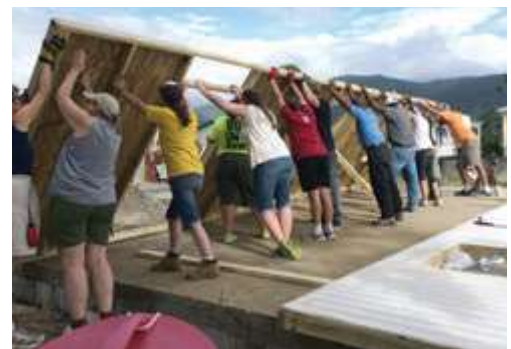
Missionary Impossible volunteers are putting up the first exterior wall of the house for Shaniqua, the single mother whose house burned down in 2011.
