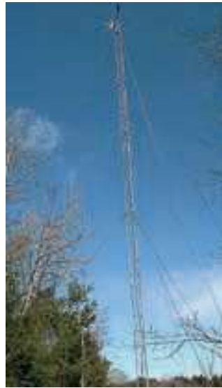
The Charlestown company has purchased a wind tower and is disassembling it and moving it to repurpose it as their new radio station tower.
