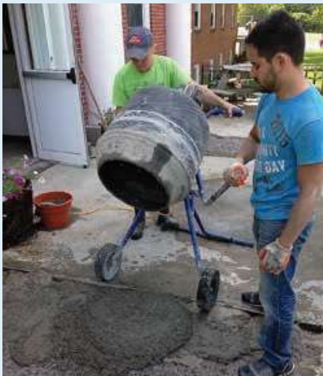
Volunteers converged on the campus of Union Springs Academy during Renovation Week to help with the much-needed renovations.
