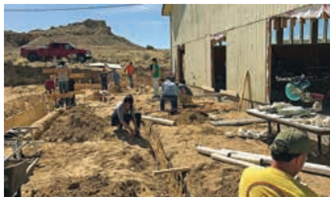
Volunteers hard at work on the construction project to add to the existing gymnasium
