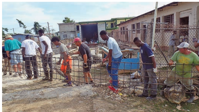
Greater New York Academy students and other workers move rebar (a steel reinforcing rod used in concrete).
