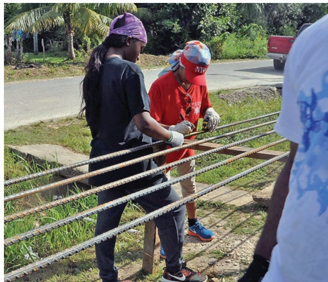
Karis McGregor and Alise Renaud, Greater New York Academy students, mark rebar at the construction site.
