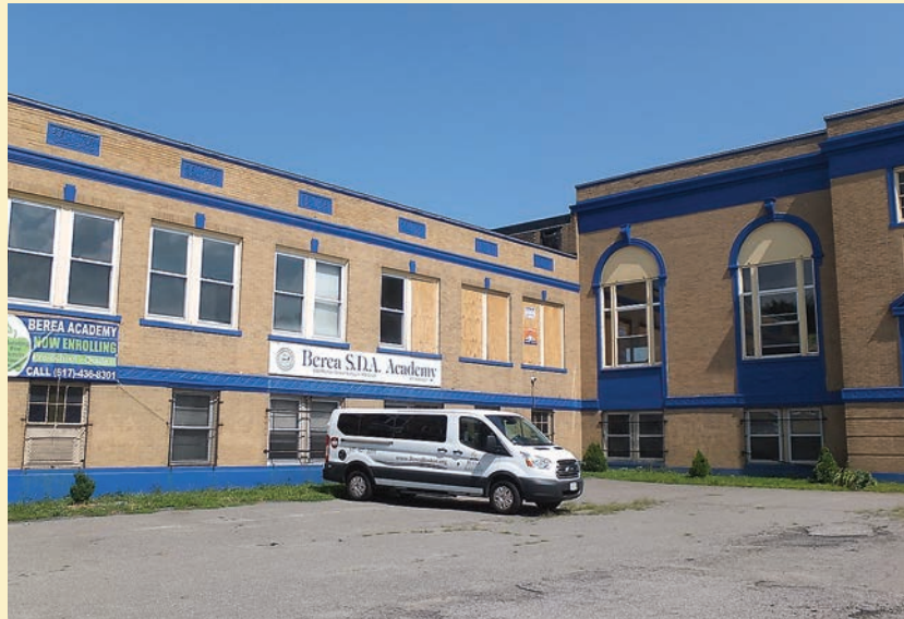
Windows boarded up are the only outward signs that a fire causing about $200,000.00 in damages occurred at Berea Academy in Mattapan, Massachusetts.
