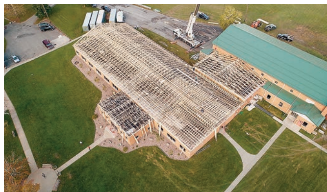
An aerial view of the construction for the new roof on the Clyde Newmeyr Administration Building.
