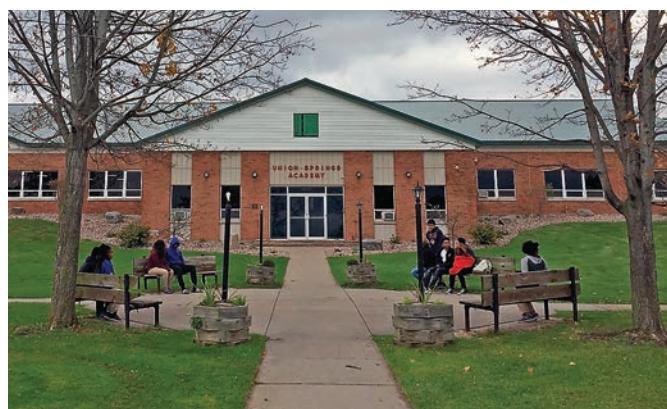
The academy classroom wing is now covered with the new pitched roof.
