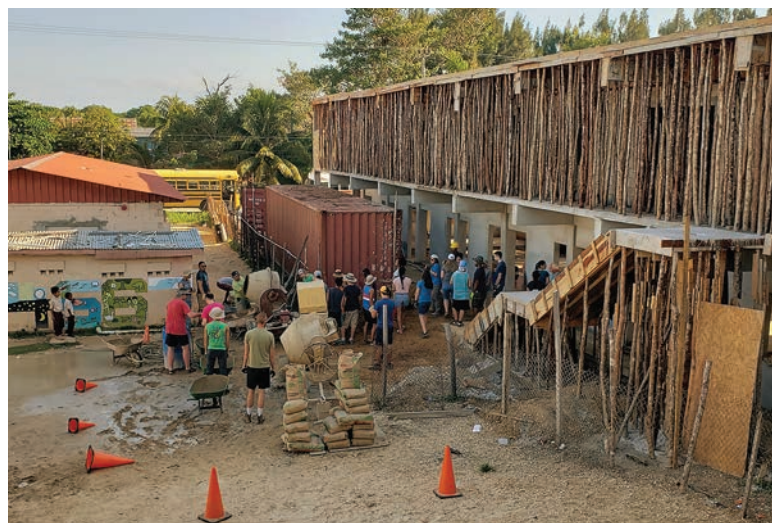
South Lancaster Academy students at the construction site gather sand to mix concrete to pour on interior floors and they also get ready to paint walls.
