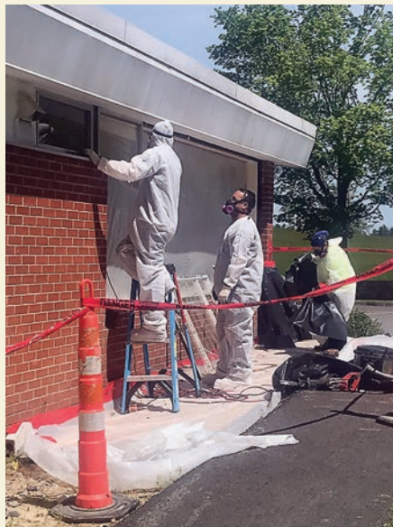
Workers install new double-paned, energy-efficient windows in the South Lancaster Academy building.
