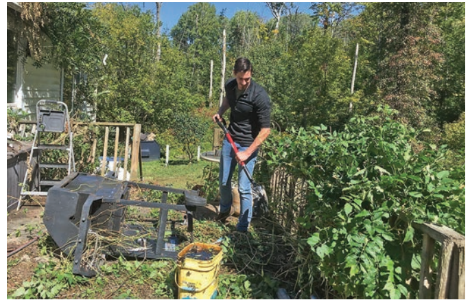
Zechariah Musselman, Randolph church senior pastor, works on the overgrown back deck.
