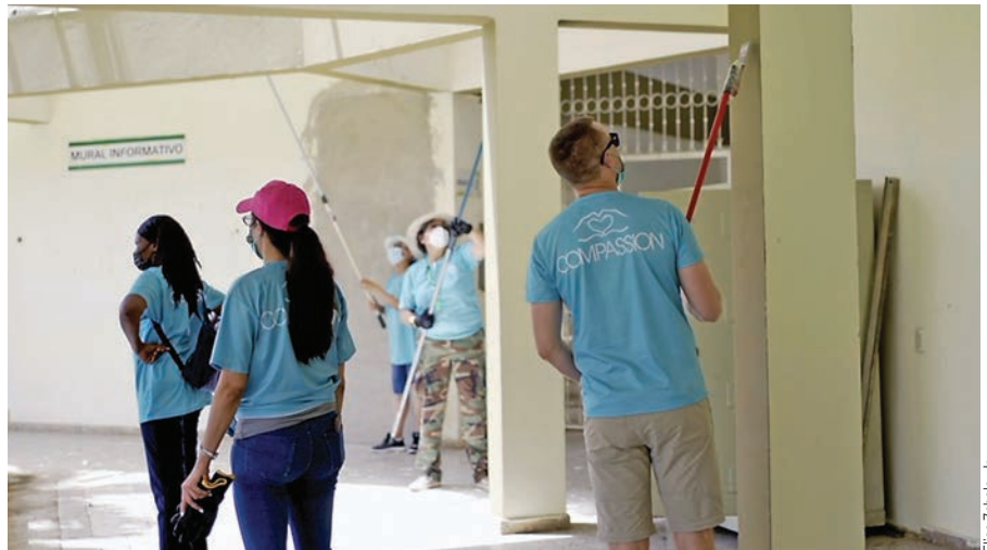
Volunteers at work scraping paint off the walls of the Dominican Adventist University administration building.
