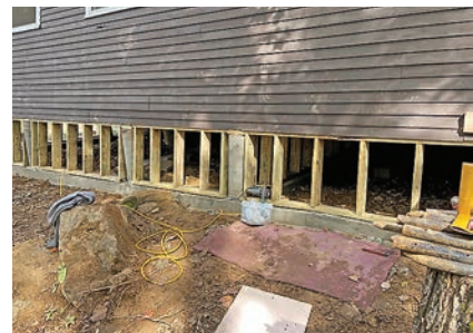
The Maranatha crew saved Camp Lawroweld’s old crafts building from eventual collapse by shoring up the foundation on three sides.
