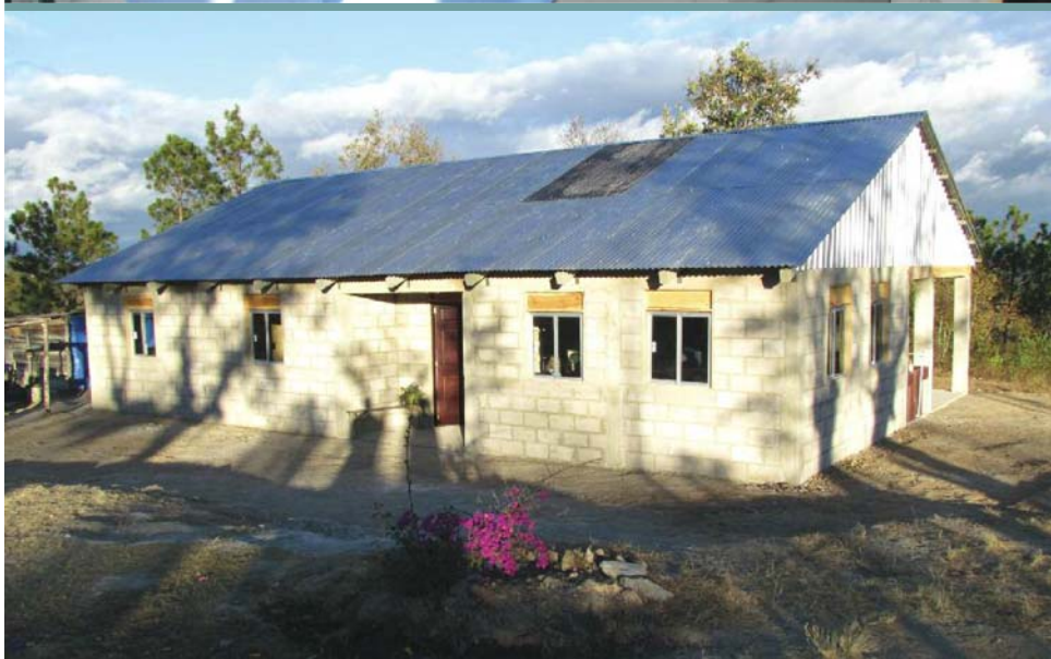
Top: Walls going up in the new home under construction with Goya's old home in view.
