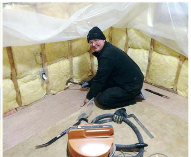
Tony Budzik, pastor, works hard at repairing the church walls during the day, and in the evening teaches Bible prophecy at the "Revelation of Hope" seminar.
