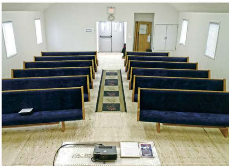
A work in progress, the newly-installed subfloor in the sanctuary awaits the installation of carpet at the Adventist church in The Pas, Manitoba.
