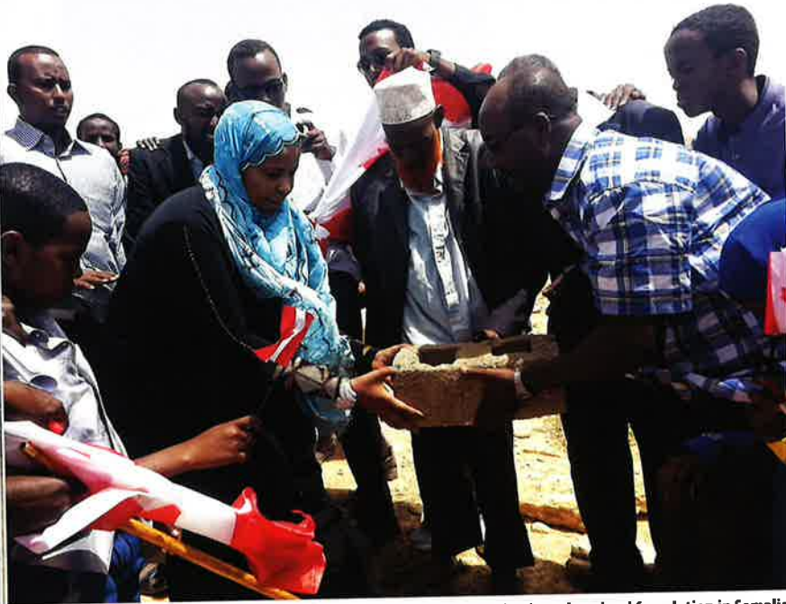
Zainab Mohamoud of Red Deer helps out with first brick going into the school foundation in Somalia. Mohamoud was on hand to see the school go up in six weeks this past summer.
