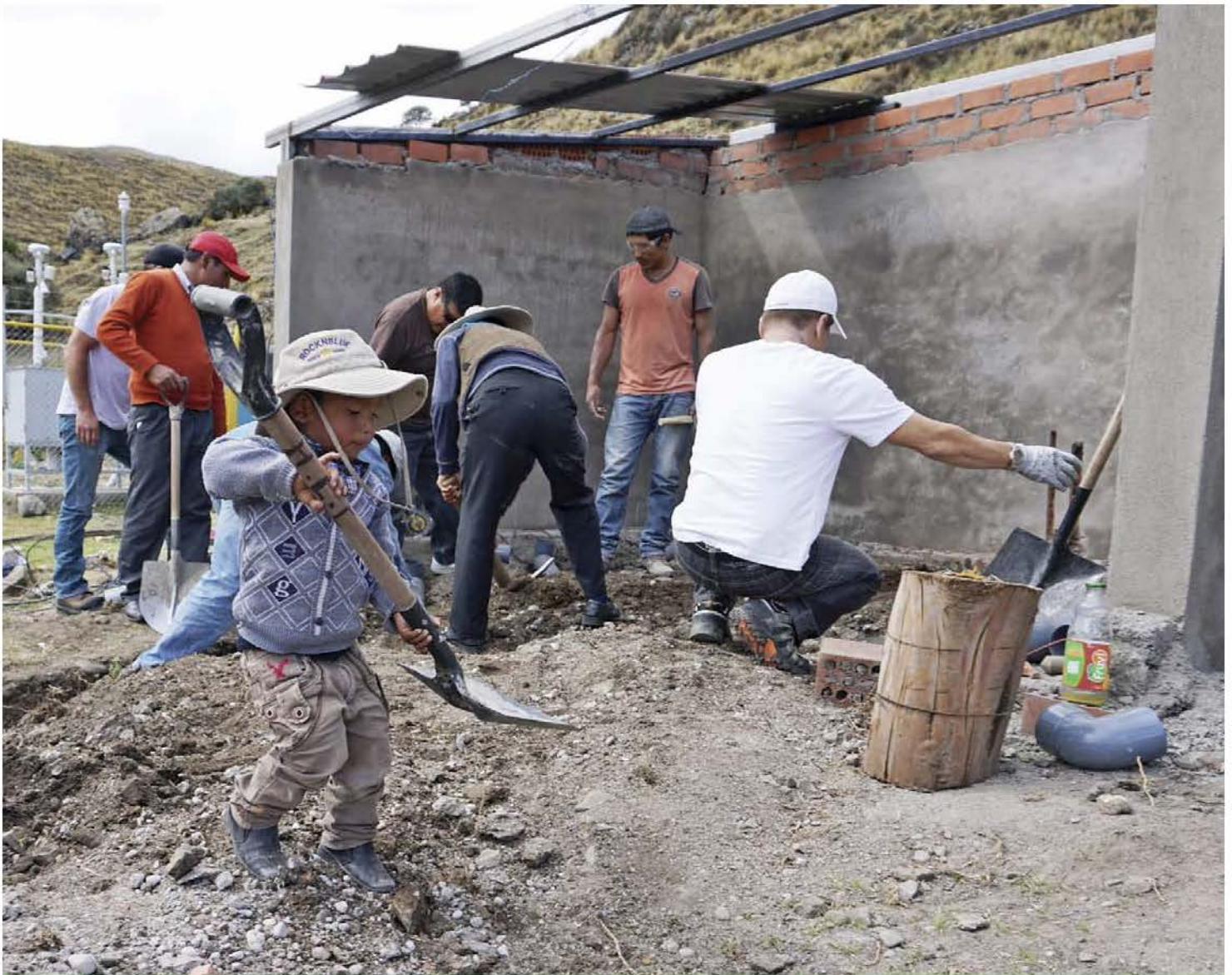
► A young Peruvian boy pitches in to help the Hamilton, Ontario team rebuild the school's bathroom facilities and septic system.
