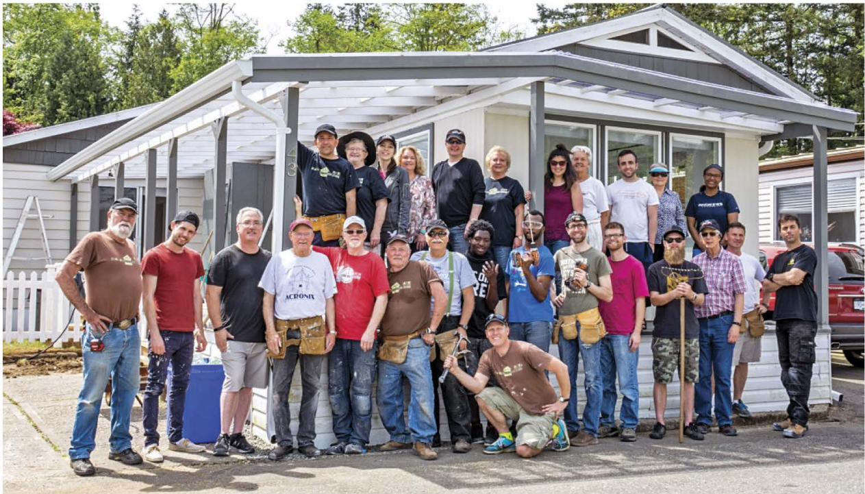
Extreme Home Repair volunteers in front of the manufactured home they renovated, inside and out, over a two-week period.
