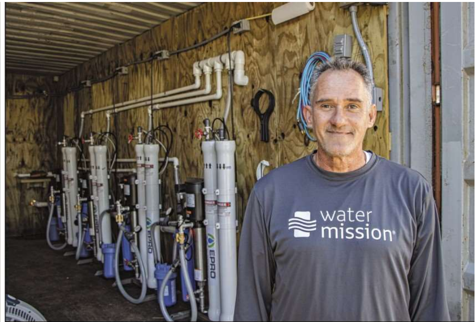
Wayne Hall shows the water filtration system in the Bahamas.
