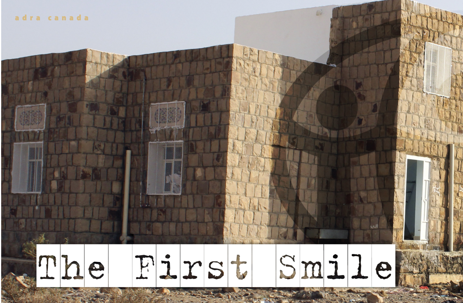
Photo above: Repair work being completed on a health facility in Yemen. Inset, opposite page: Mahmoud before and after his surgery; a doctor working with the ADRA project.
