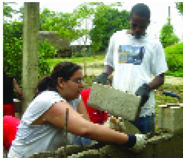
Juniors Kayla Alcott and Joshua Asamoa lay block walls for a new Seventh-day Adventist church in San Pedro.
