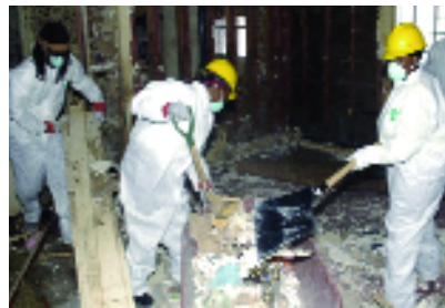
Volunteers had to wear protective clothing and masks while they gutted the damaged homes.
