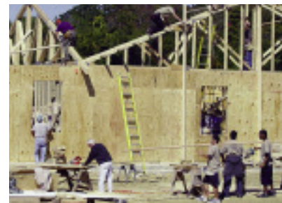
Volunteers have made the past three Arise and Build projects successful and are requested again to help erect a new building on September 23 for the Everett church.
