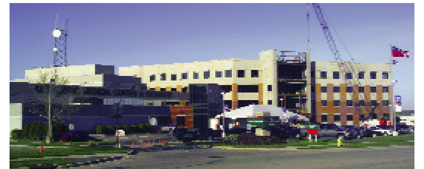
Kettering Medical Center-Sycamore's expansion will feature a spacious front lobby with retail shops, a pharmacy, and refreshment center. A sleep center, breast evaluation center, wellness education, patient registration, lab, and outpatient services will also be housed in the new facility.
