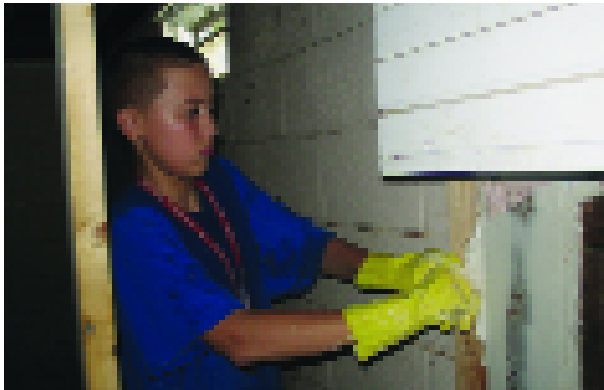
Senior Matt Brown helps pull down destroyed drywall from an affected home in Shelby, Ohio.
