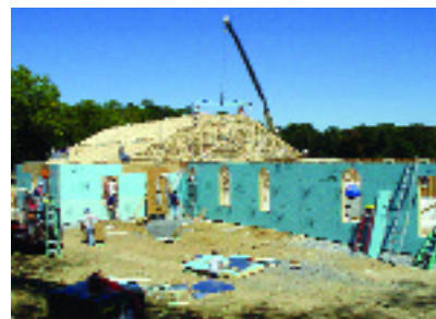
By the end of the day, all outside walls were in place, trusses were being set, and the church was taking shape.
