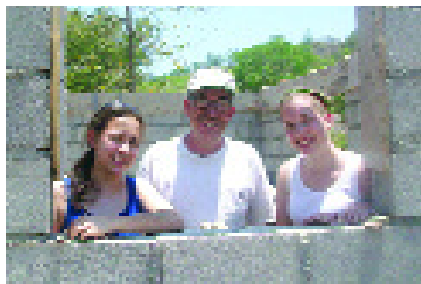
Kylynda Bauer ('09), former parent Bill Jackson, and Jennifer Calhoun ('10) stand in a partially finished home on a recent mission trip to Honduras.
