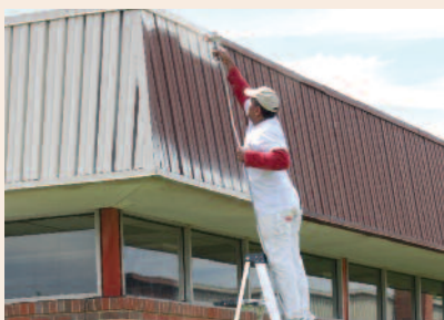
Painting the exterior of Takoma Academy's building is just one of many exciting changes taking place at the Takoma Park, Md., school.
