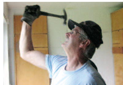
Ed Cale, an alumnus and parent, continues in the footsteps of Blue Mountain Academy's pioneering supporters as a volunteer in a recent renovation project.
