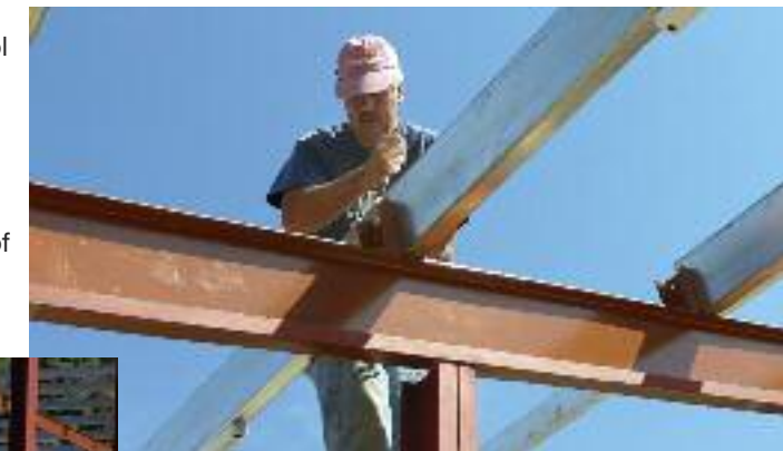
Spencer Hannah, SVA principal, works on the roof of a new school in Lesotho.
