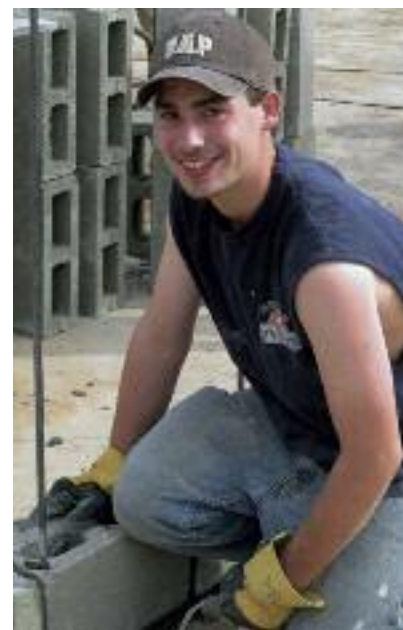
The author lays bricks to build an elementary school in the African country of Lesotho.
