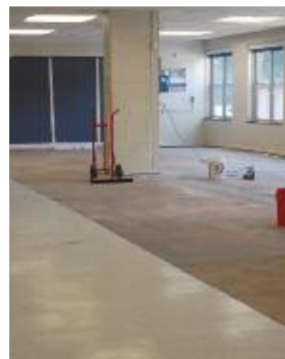
The partially retiled cafeteria floor will be completed by the time school re-opens.
