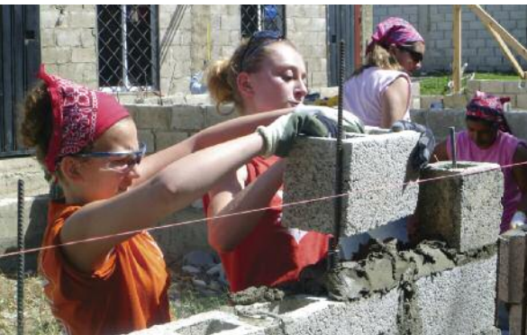
Amanda Linzau, Gabby Cook, Amber Dahabura and Shannon Injety work tirelessly on the construction of the school building.
