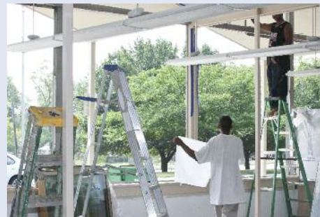
Workmen replace all of the glass at the front of Sligo Adventist School.
