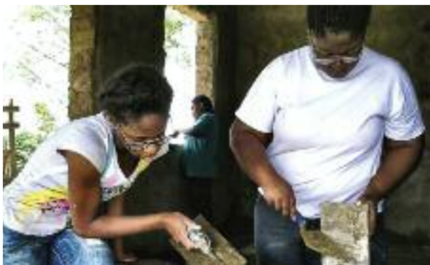
Freshman Briana Marshall and junior Ashley Laing help build an administration building at the Havilah Orphanage in Tanzania.
