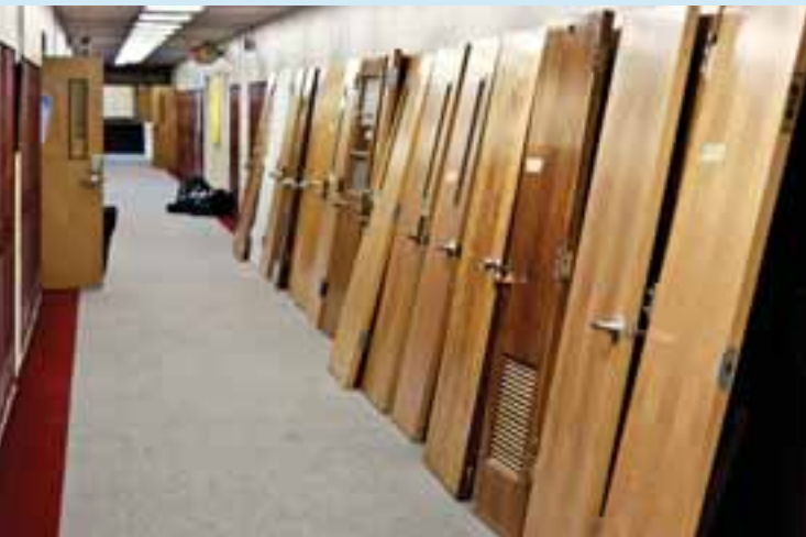
As part of Takoma Academy's continuing renovation process, classroom doors will be refinished.
