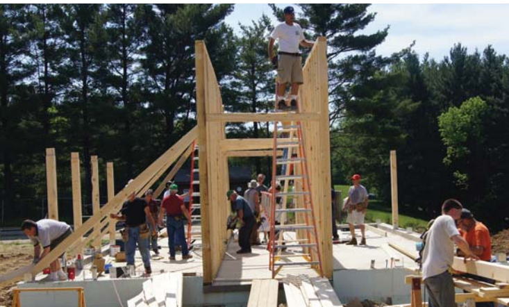
Manfest attendees lend their muscles to help construct a new bathhouse for Camp Mohaven in Danville.
