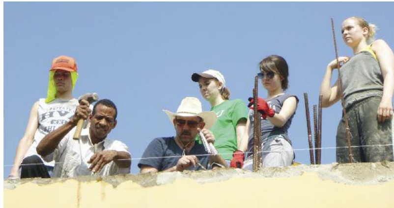
Students (back row) Derrick Dye ('14), Cassondra Harris ('14), Kabrina Perkins ('14), and Valerie Wyatt ('15) work with parent Paul Shingleton (in the hat) and a local church member on a wall of the new school auditorium in La Isabella, Dominican Republic.
