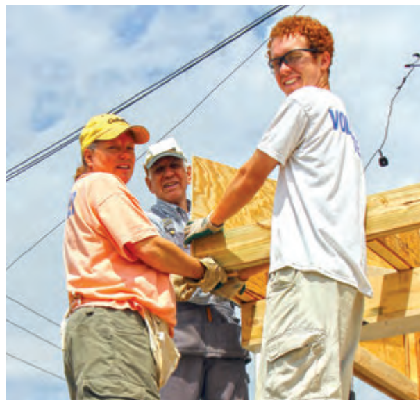
Maranatha volunteers Lee Achenback (back) from Takoma Park, Md., works with Louann Kratzer and her son, Jeff, from Georgia, to build a porch for a staff house.
