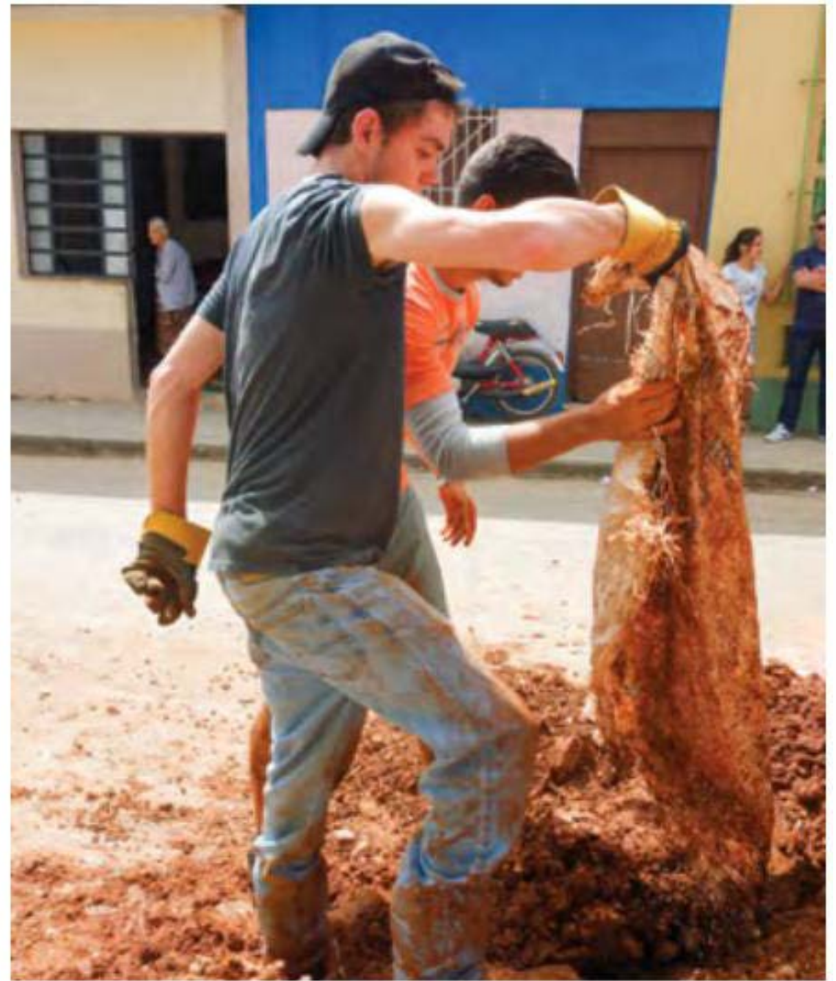
Home school student Elliott Ackman helps a Cuban worker carry dirt from a building site.
