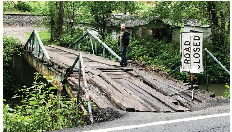
A flash flood in 2015 destroyed this bridge, making it nearly impossible for 13 Pigeon Creek families to get access to food and medical care.
