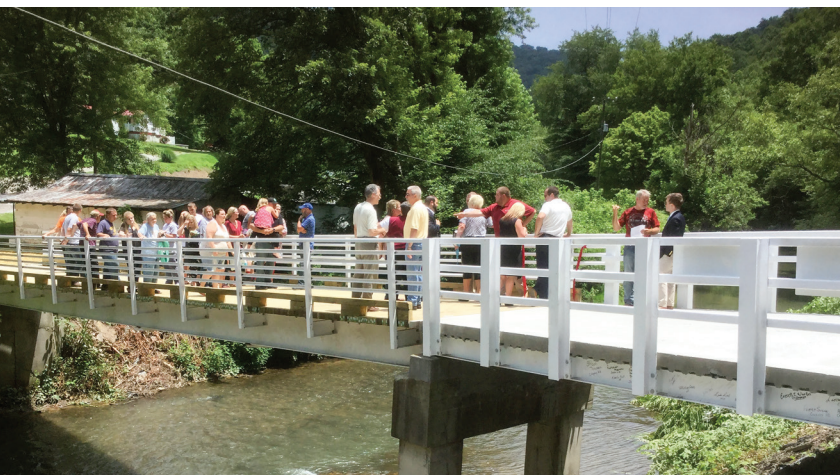
In 2017 with the help of Adventist Community Services, volunteers constructed a 90-foot bridge, giving full access to and from the Pigeon Creek neighborhood.
