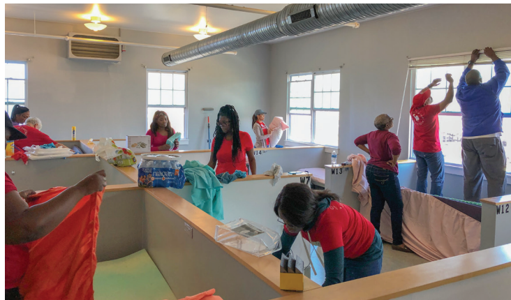
Takoma Park church volunteers clear and prepare a 15-bed women's shelter quarters for renovation during "Service Sabbath."
