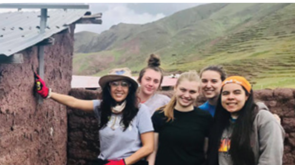
Elementary Vice Principal Judie Rosa, Izzy Touma ('22), Jackie Whitsett ('20), Erin Beers ('20) and Isabele Arteaga ('19) take a break after installing solar panels on a one-room adobe home that never before had electricity.
