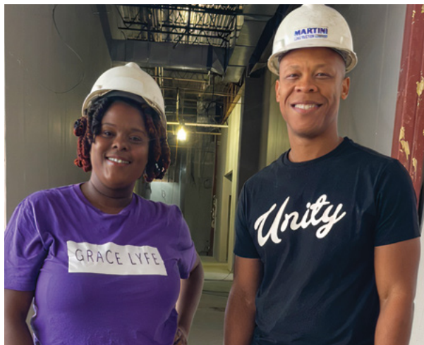
Pastors Regina Johnson and MyRon Edmonds tour the new Grace Community building site.
